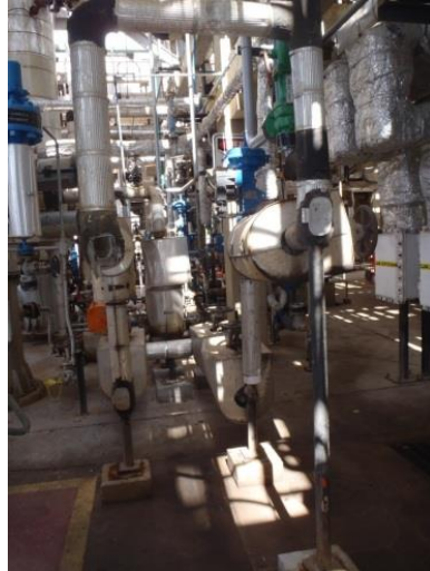
Figure 2: Portions of the piping exiting the pressure vessel.
