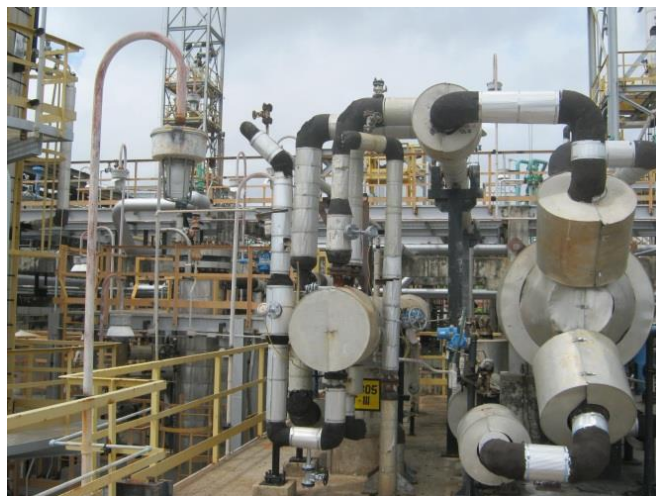
Figure 1: Overview of pipe system close to the heat exchanger.
