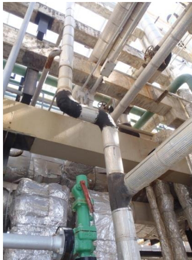
Figure 3: Pipe detail near the heat exchanger.
