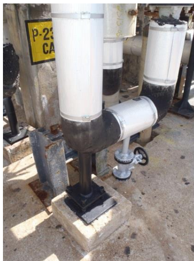
Figure 4: Detail of one of the pipe brackets, next to the heat exchanger.
