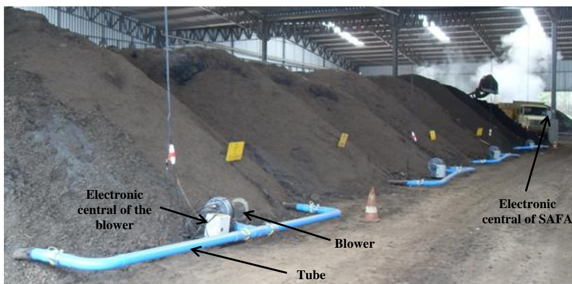
Figure 3 - SAFA installed in the compost shed.
