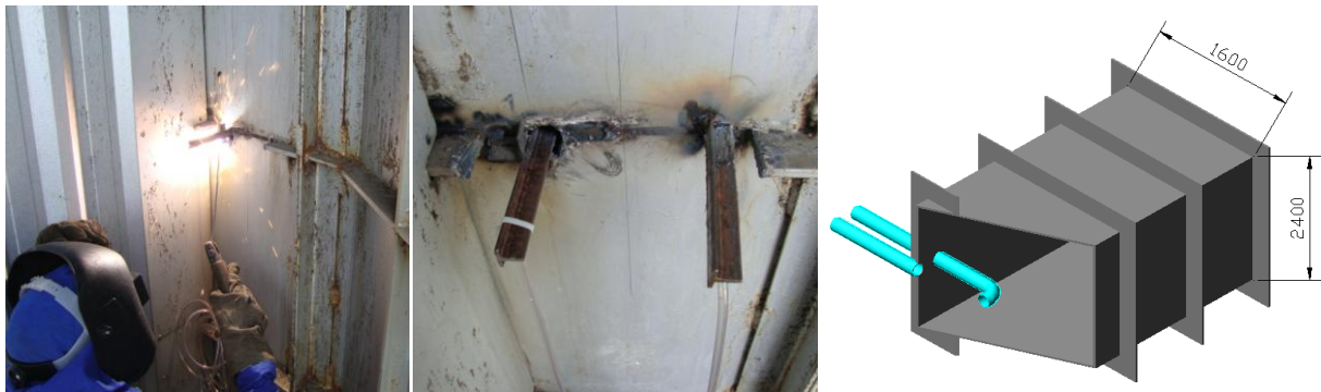
Figure 4. Pitot tube installation – Primary Air Duct
