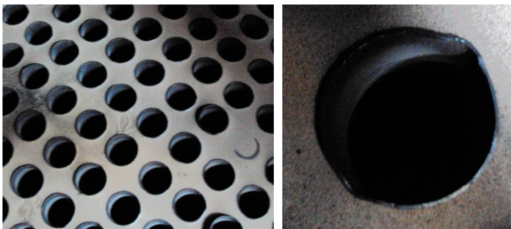
Figure 12. Preheater Tube Bank after 792 Operation Hours.
