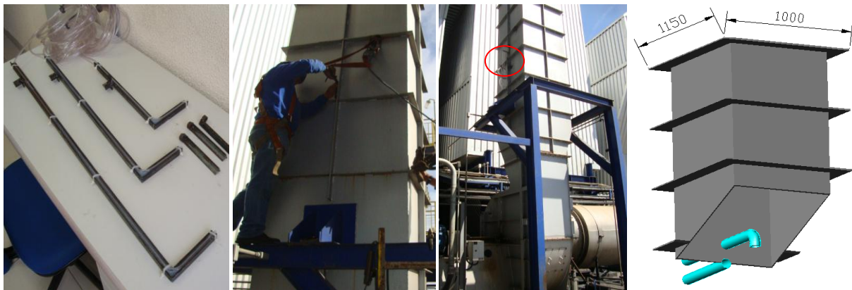
Figure 3. Pitot Tube Installation – Secondary Air Duct
