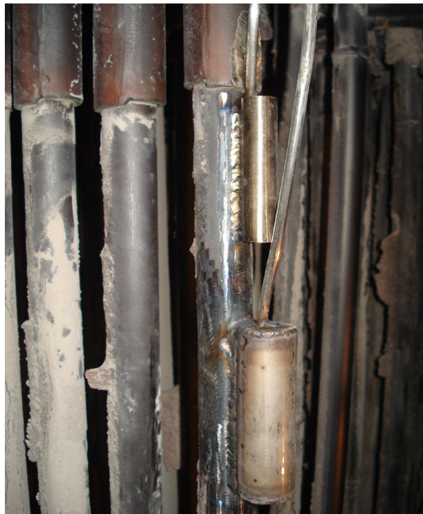
Figure 5 - Surface temperature sensors installed on a final superheater tube.
