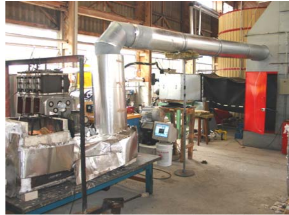
Figure 6. Induced draft furnace connected to the dryer
