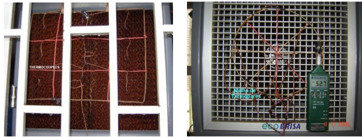
Figure 6. Thermocouple installation at the supply tested and the exhaust face of EAC showing thermohygrometer used.
