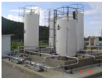
Figure 8. tanks of the LAMP
