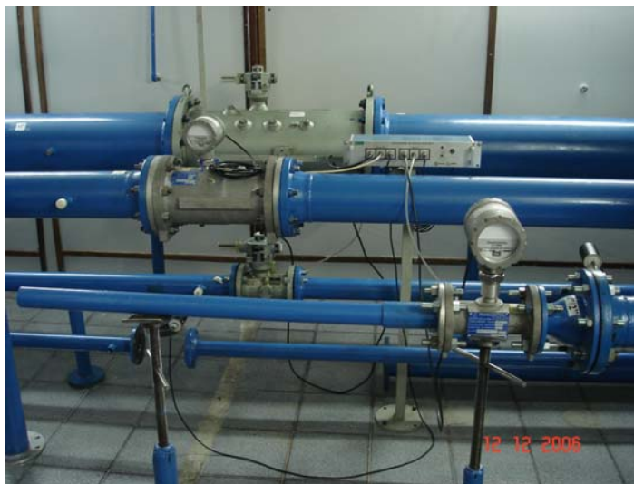
Figure 1. Overview of the turbine calibration facility.
