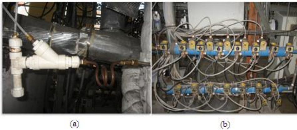
Figure 3. Pressure measurement system: (a) filtering and cleaning system; (b) solenoid valves
