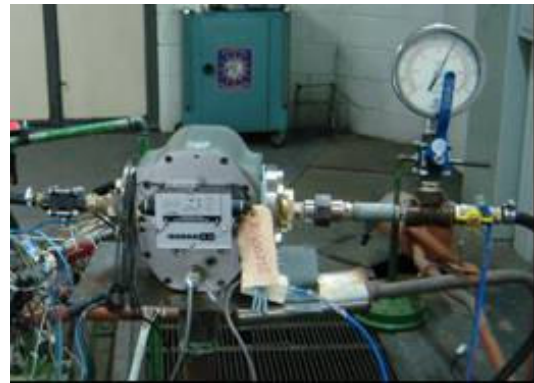
Figure 2. CNG Flowmeter coupled to system
