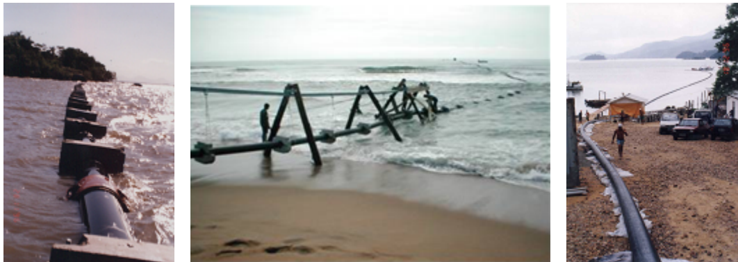
Figure 1: Use of HDPE for submersed water distribution pipes.
