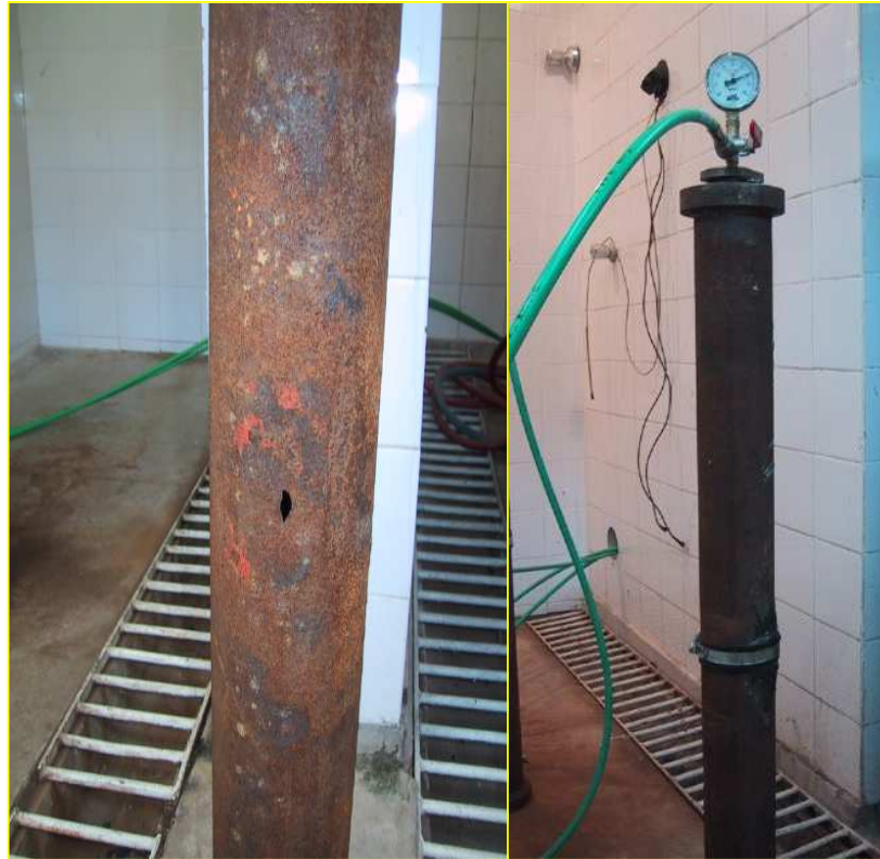
Figure 11: 3,5" diameter, schedule 20, 1000 mm length pipe with real corrosion defect before and after repair.
