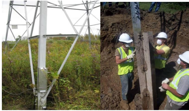
Figure 6: NDE System During Inspection of Transmission Line Stub Angle (left) and Actual Excavation and Inspection (right)
