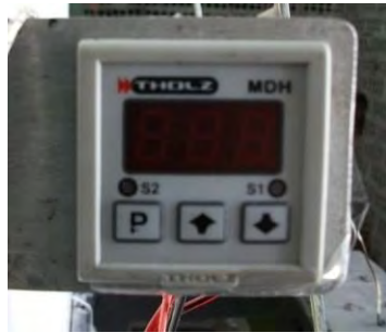
Figure 5. Digital controller/indicator of temperature
