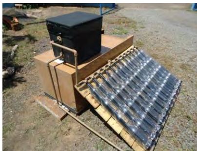
Figure 11. SWHS installed (Author, 2013).
