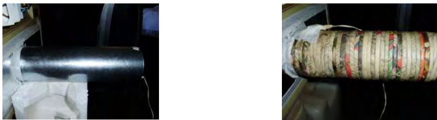
Figure 2 – Digital thermometers installed in the inner and outer side of the ducts.
