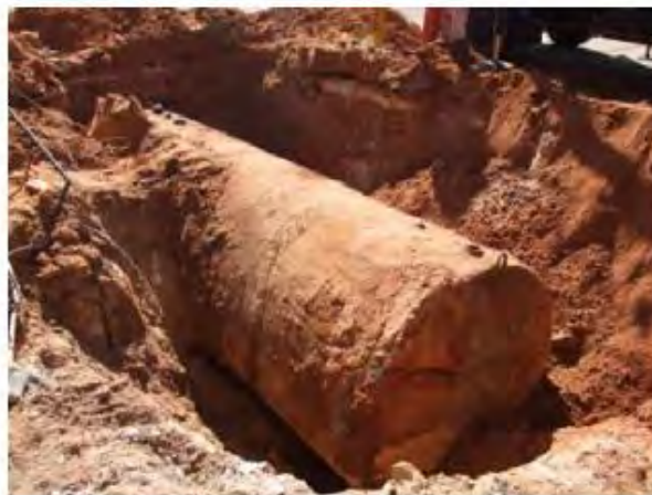
Figure 7. Corrosive state of a buried tank used for the storage of liquid fuel at a gas station in Natal (RN).
