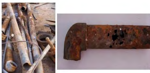
Figure 5. Details of the status of pipe used in gas stations.
