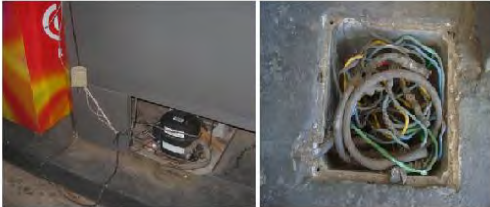
Figure 6. Wiring and electrical system found inappropriate in a retail fuel station.
