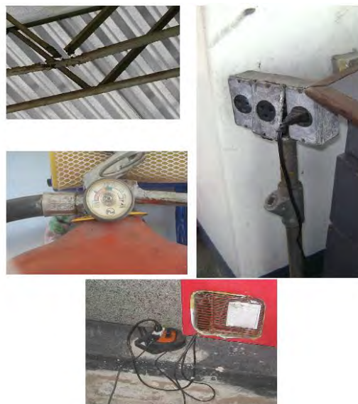
Figure 4. Details of the metal structure of a retail fuel station; the charge level of a fire extinguisher located in a retail fuel station; electric system found in a retail fuel gas station and electric system found in a gas fuels reseller.
