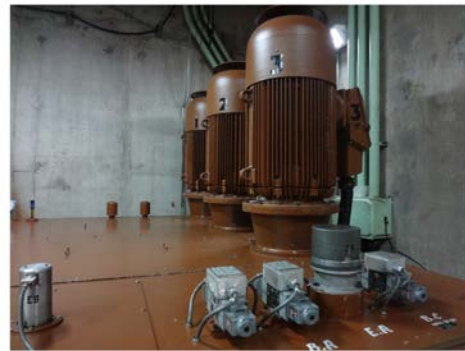
(b) Pressurization pumps drivers
