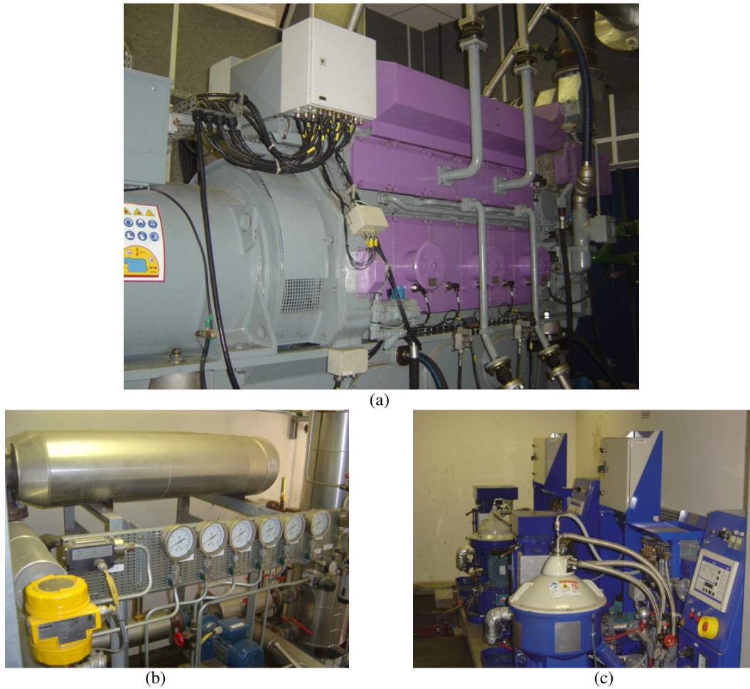
Figure 1. Diesel Engine (a) and auxiliary equipments (b,c)
