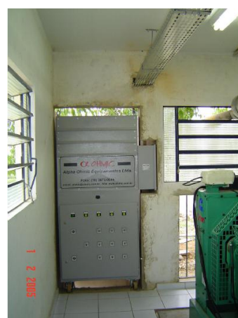
Figure 3. Resistive load Bank
