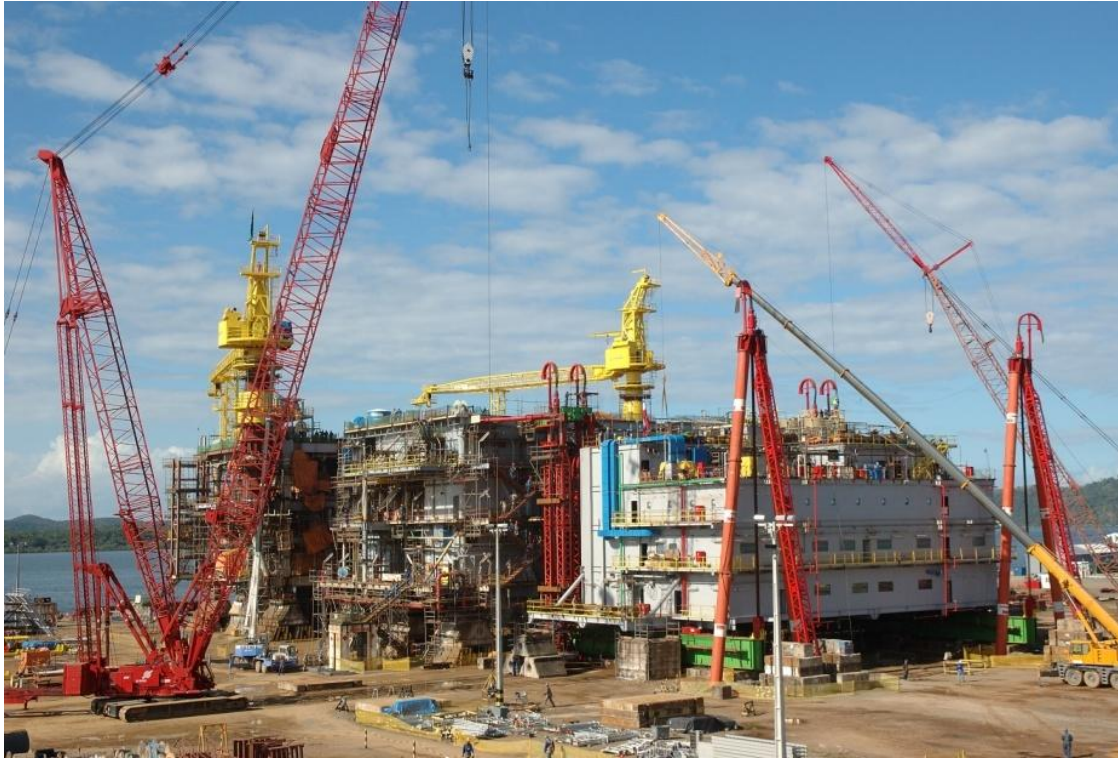
Figure 1. Construction of three modules for PRA-1 Offshore Platform. Photo courtesy of Odebrecht, Luciano Andrade.
