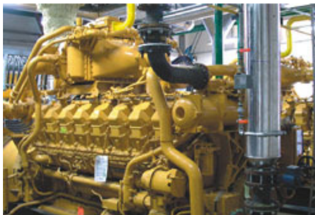
Figure 1. Picture of the cogeneration plant motor generator group
