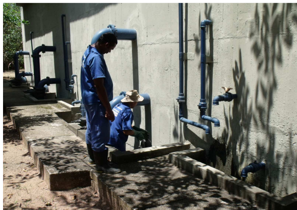
Figure 3. Sludge discharge points in the UASB reactor
