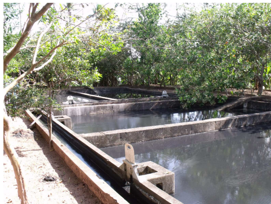
Figure 4 – Sludge sand drying bed
