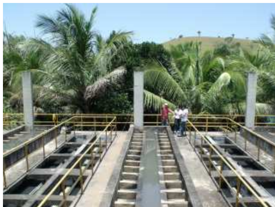
Figure 1. The Rio Formoso sewage treatment plant
