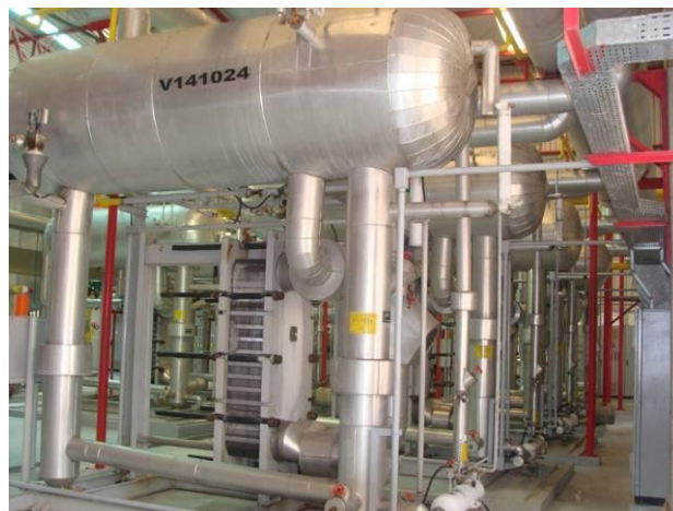
Figure 2: Cooling units / NH 3 evaporators
