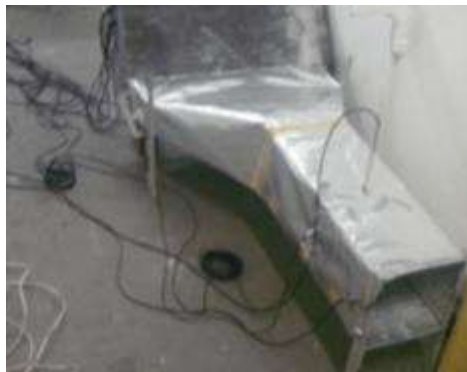
Figure 3. Instrumented evaporator Air duct
