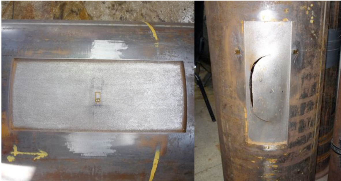
Figure 1. External defect of a specimen without composite reinforcement, also showing the strain gage and burst pipeline
