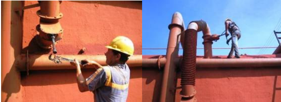
Figure 6: Operational of opened of valves of the heat exchangers device.
