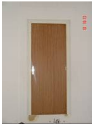
Figure 4. Installed view of Door 3.
