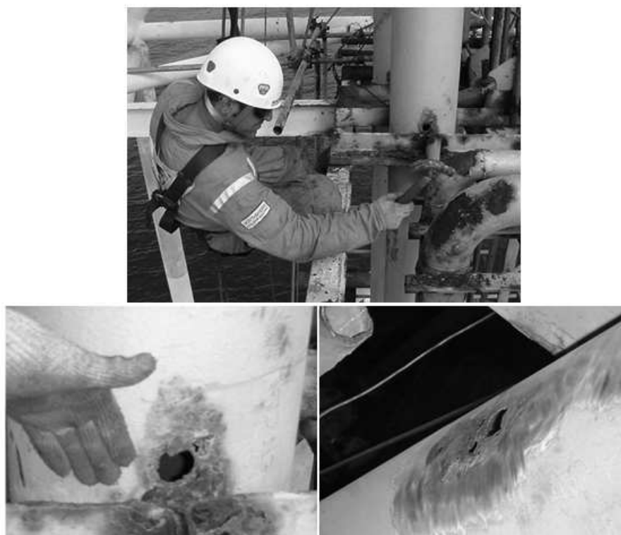
Figure 1. Corrosion damage in produced water pipelines
