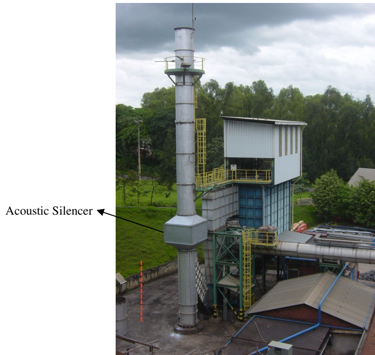
Figure 3. Noise silencer for exhaustion system
