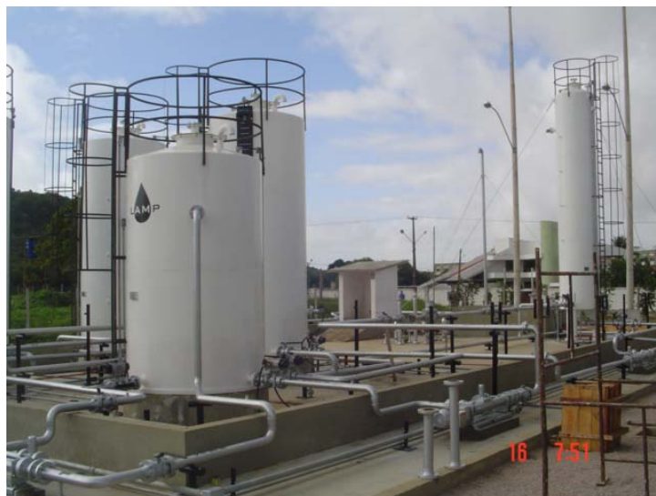
Figure 1. A view showing the (LAMP) Laboratory Plant
