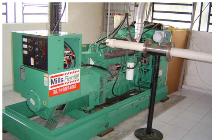
Figure 1. Diesel engine and electrical generator system.
