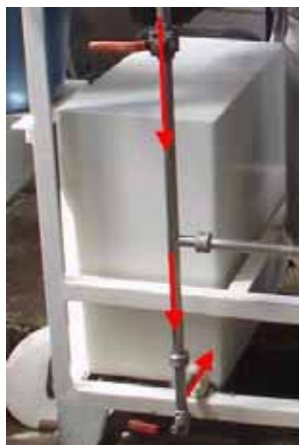
Figure 13. Inlet of the heat exchanger.
