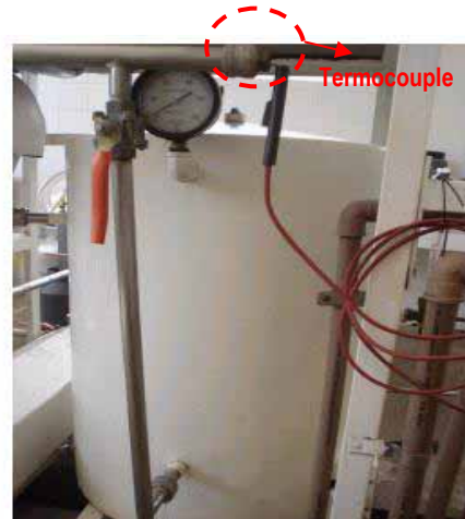
Figure 8. Termocouple installed in the boiler.
