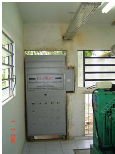
Figure 4. Bank of electrical load with capacity of 150 kW.
