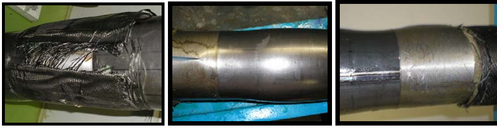
Figure 17. Fracture and delamination of the repair, as well as strangulation of the steel wall and less deformation at the sewed region of the pipe (i.e. the welded meridian)
