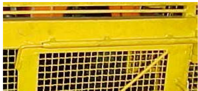
Figure 5. OP-40 – (a) Door lock; (b) Door rail closed.
