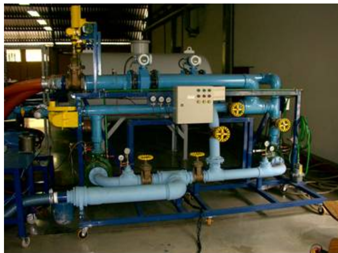
Figure 5. Pumping system developed to provide several turbine pressure and flow conditions.
