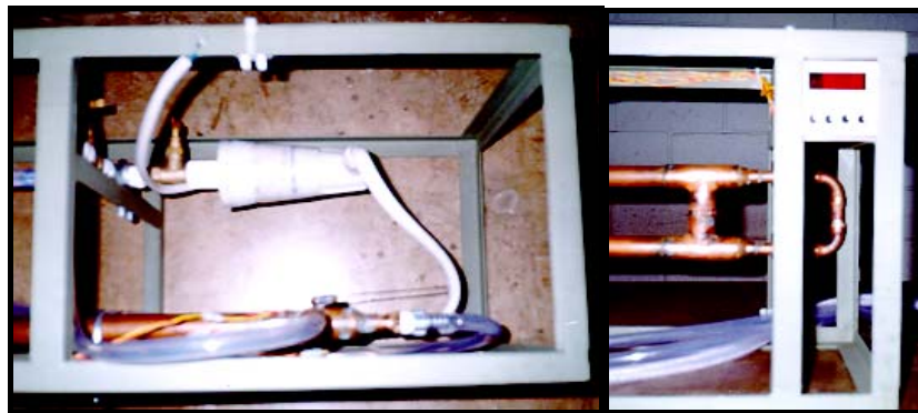
Figure 2. Rack Details and thermometer installation.
