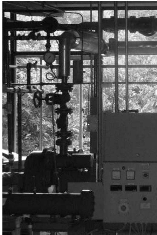
Figure 1. Control valve, turbine and condenser (bottom) setting.
