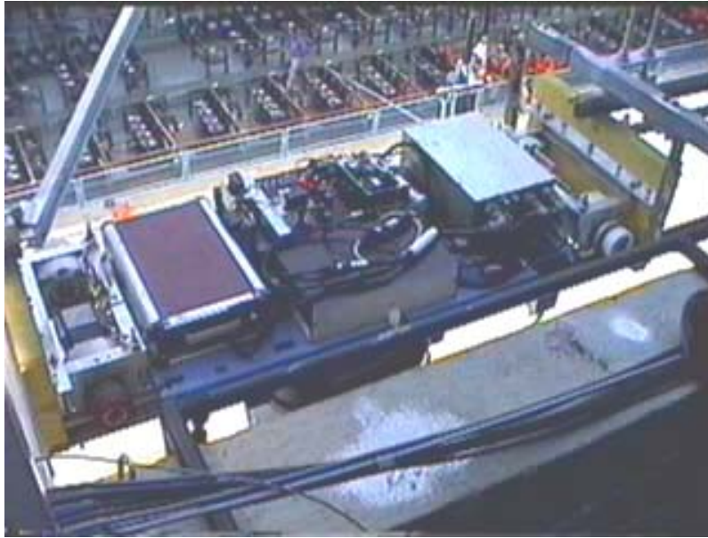
Figure 7. Trolley with onboard equipments on site.
